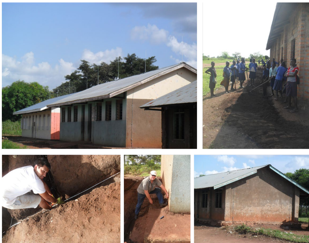
Figure: Lightning protection system installed at the Runyanya Primary School in Kaburasaho, Uganda. This is one activity that Zhang has been involved with over the years as an external participant of the UCAR Africa Initiative (photo taken in 2017).
