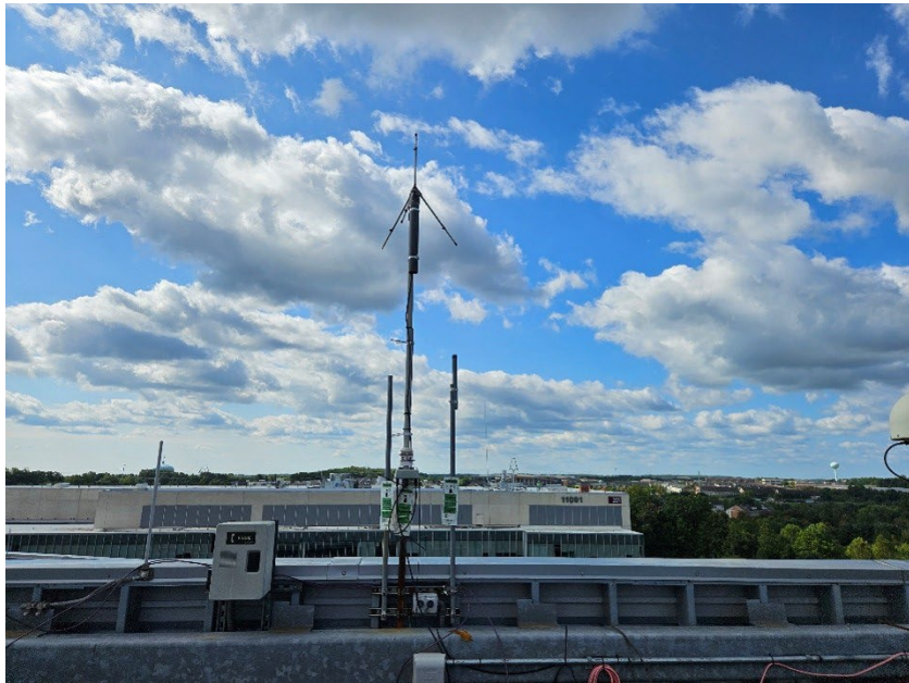
Figure: The VHF antenna (center) for this sensor at JHU APL. The proposed new sensor relocation site is on the roof of the building in the background. Photo credit: Joseph Patton
